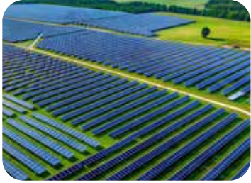
Renewable-energy power plants
